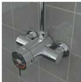
Exposed valve - top outlet
