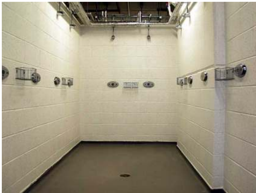
Rada Sense digital showers have been installed in all of the shower areas in the Millennium Stadium players changing rooms.
