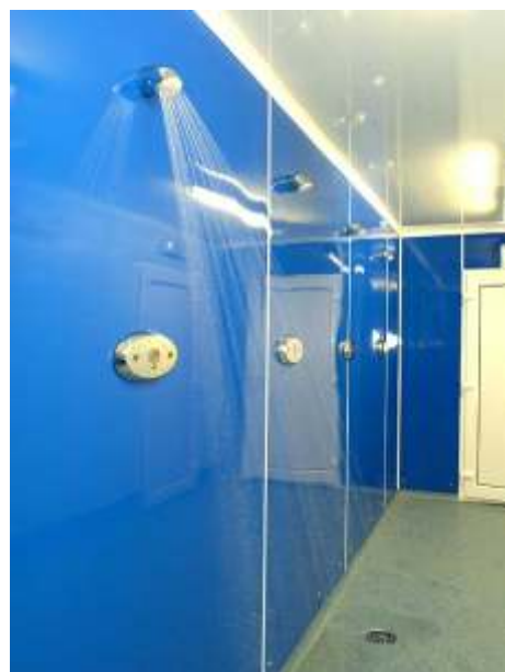
The Rada Sense controlled showers in the North Wirral Soccer Dome.
