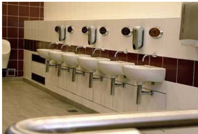
1: One of the upgraded washrooms in the Royal Liver Building, Liverpool featuring Rada Sense digital water control systems to control water supplies to all of the wash hand basins.
