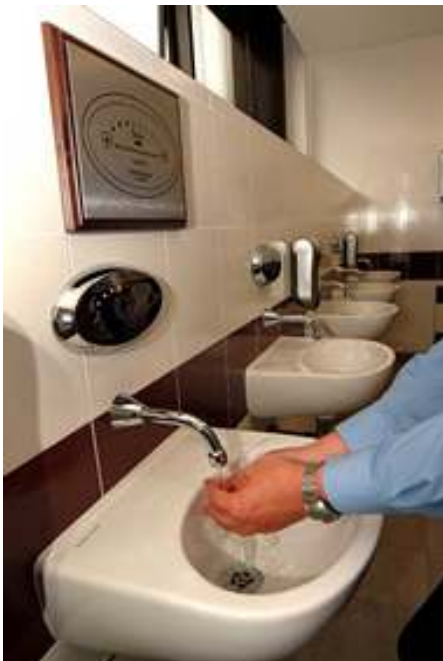
2: Rada Sense units control both the water on/off operation at each basin as well as the water temperature control..
