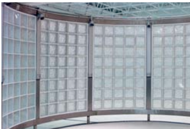
Interior of poolside shower feature with Rada-Presto PA400s shower panel assemblies
